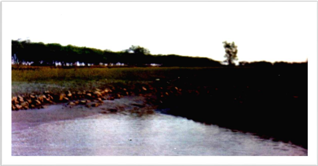
Performance of JGT on erosion control at Nayachara Island. [Photograph was taken 11 years after completion of work.]
